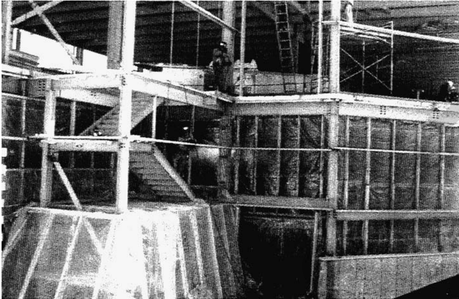
Figure 8.9 Structural steel erection for equipment mezzanine. (Photo courtesy of Gilbane Building Co.)
