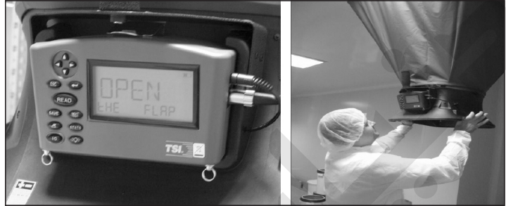
Figure 2: Micromanometer attached to the flow hood (left), measuring supply terminal with the flow hood within cleanroom (right).
