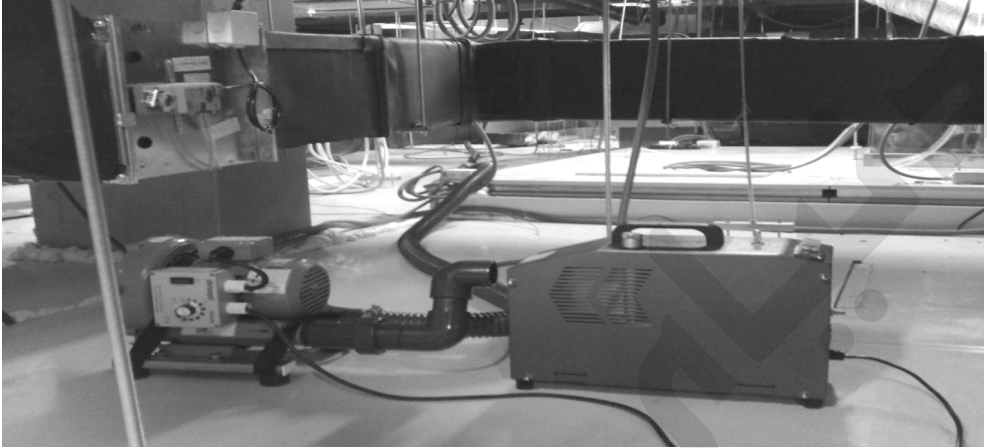
Figure 9: Connected positive injection pump and thermal aerosol generator.
