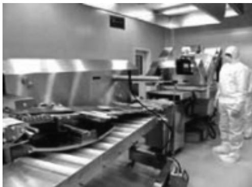
Figure 15.4 ISO 5 (class 100) clean room (courtesy of Sinteco).
