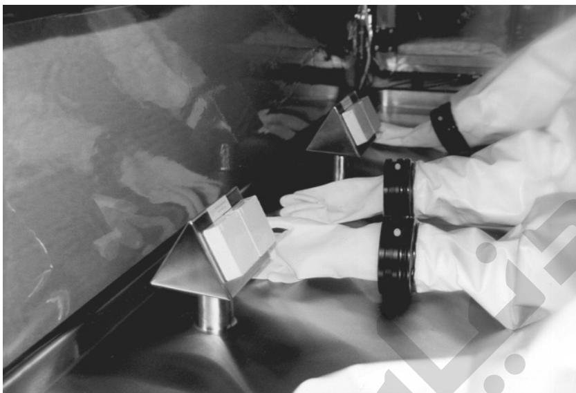
Figure 3.28 Electrical Power Sockets Fitted to a Glove Isolator. The sockets are fitted to the glove isolator in stainless steel “Christmas trees” to elevate them above any liquid spillage. (Courtesy of Astec Microflow.)
