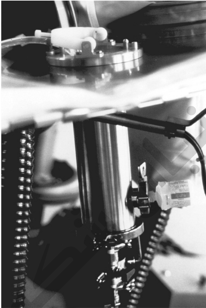
Figure 3.27 The Aseptic Connection of a Product Hose to an Isolator Using a Small RTP. In this case, the connection is through the base tray of the isolator. The stainless steel autoclavable RTP container is seen docked below the tray. The port in the tray is open, and the product hose bends away to the left of the picture. Note the hydrophobic filter fitted to the bottom right of the container. (Courtesy of La Calhène SA.)
